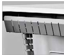
Individual metal cable tray
